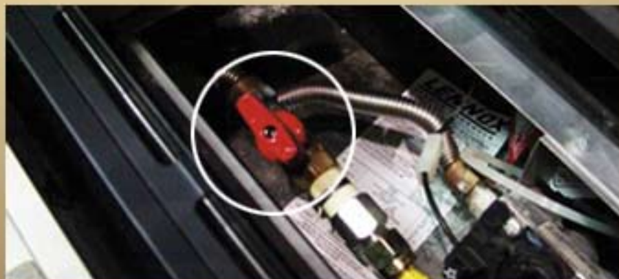
Gas supply in the ON position
